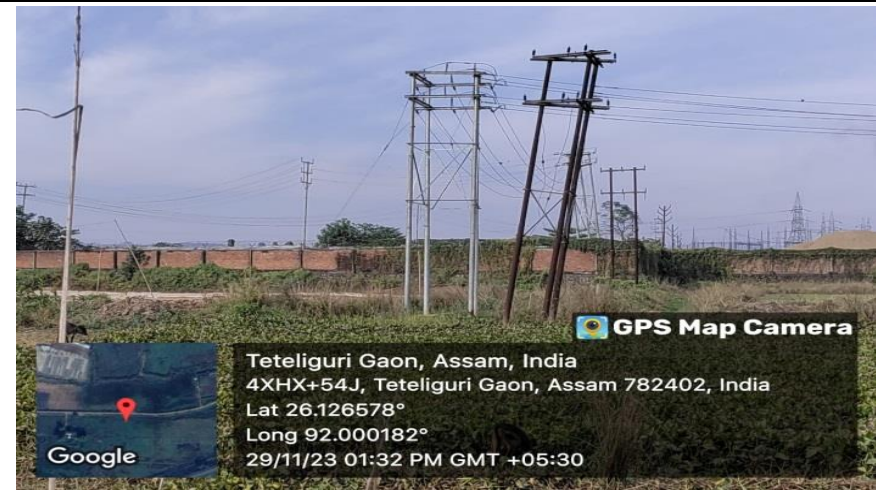
Photo Plate 8- Electrical poles required to shift during the construction of the approach road. (Ch. 450.00 mts)
