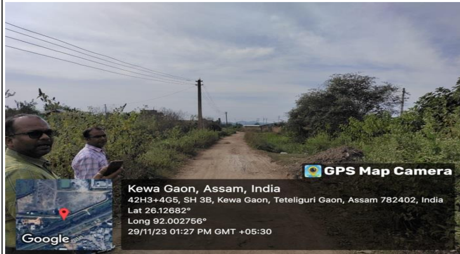
Photo Plate 5- Electrical poles required to shift during the construction of the approach road. (Ch. 180.00 mts)
