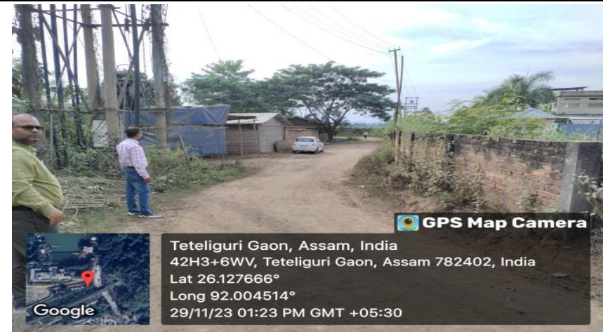
Photo Plate 4- Boundary wall need to demolish during the widening of the road. (Ch. 20.00 mts)
